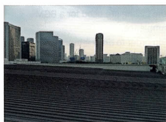
The zinc roof above Club V6 Armani was allowing too much SPL into the surrounding residences
